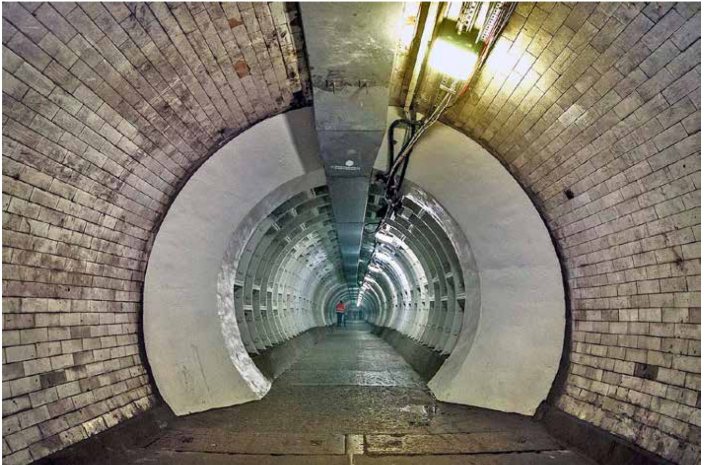
The northern end of the Greenwich foot tunnel was damaged by bombs during WWII. It was repaired using a thick steel and concrete inner lining that reduces the diameter for a short distance. Photo Andy Kirby
